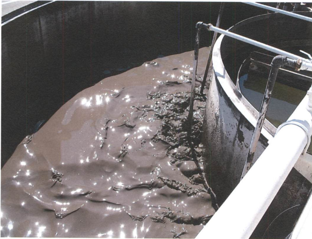
Sludge digester section of package plant.
