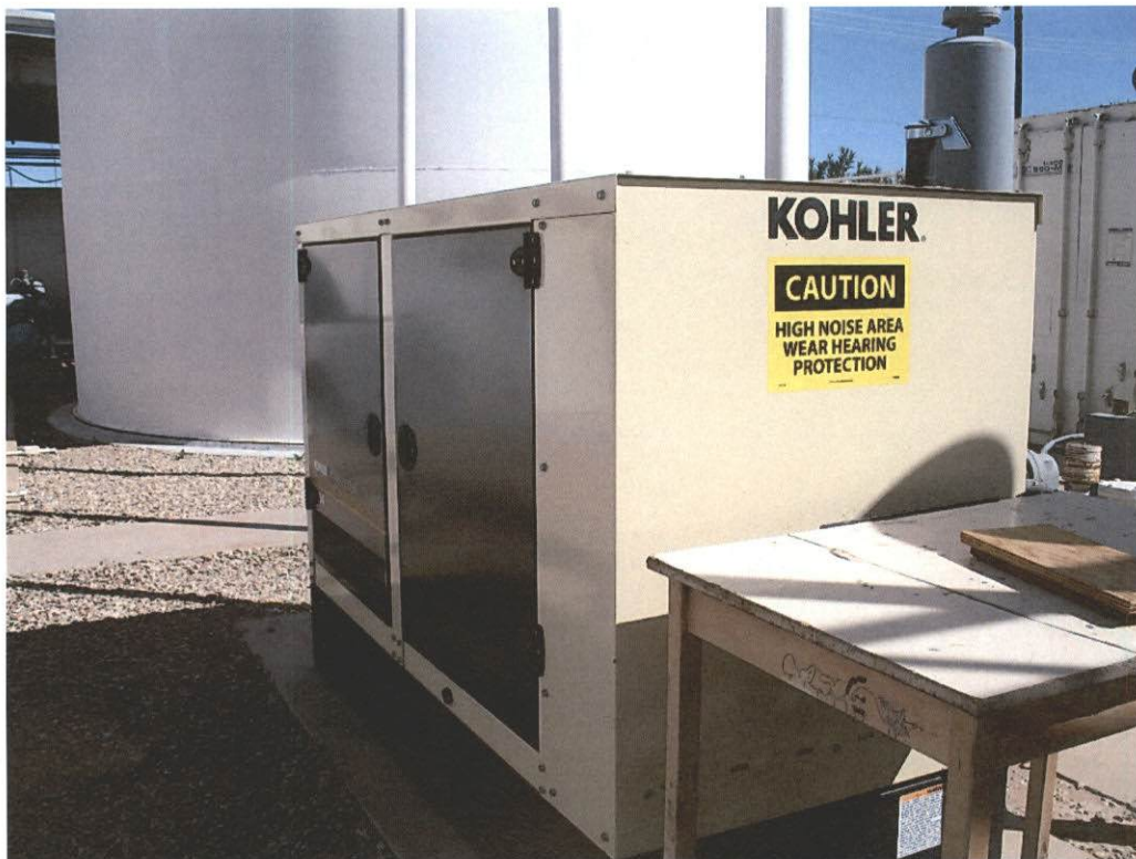
Backup power generator.
