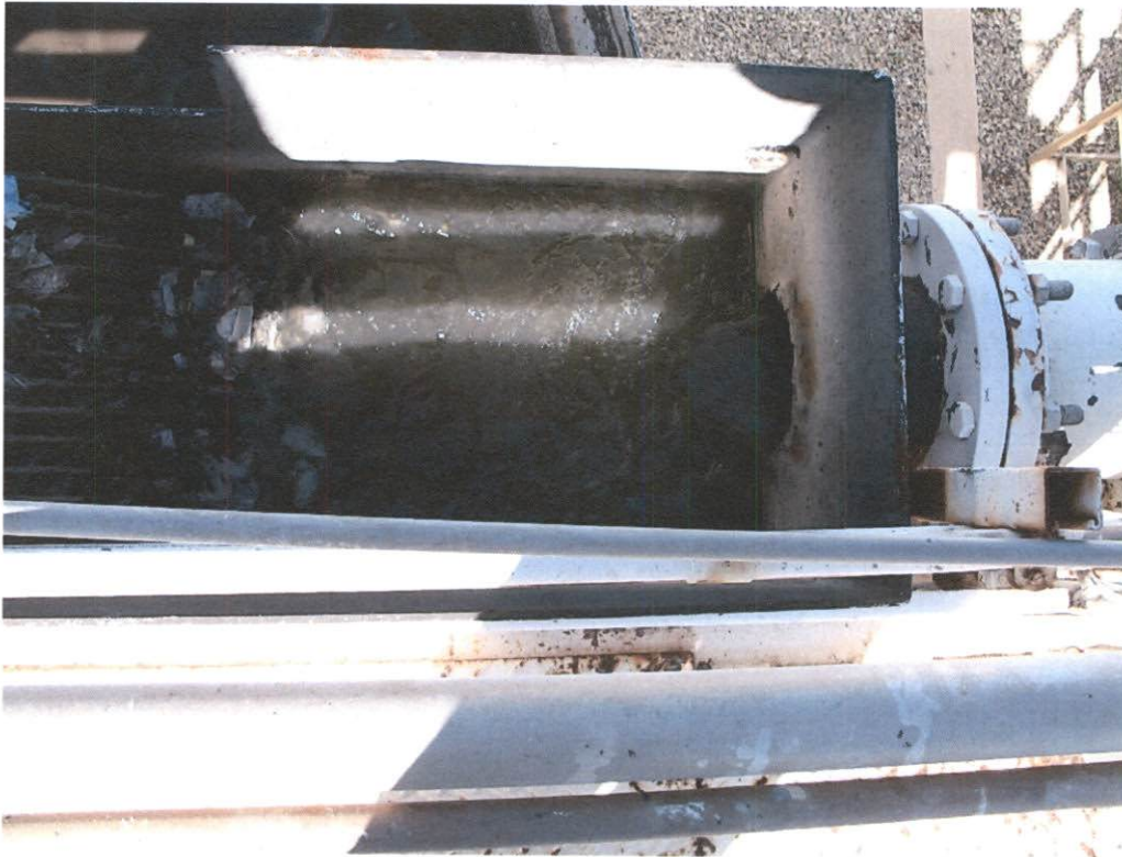
Influent monitoring location at bar screen.
