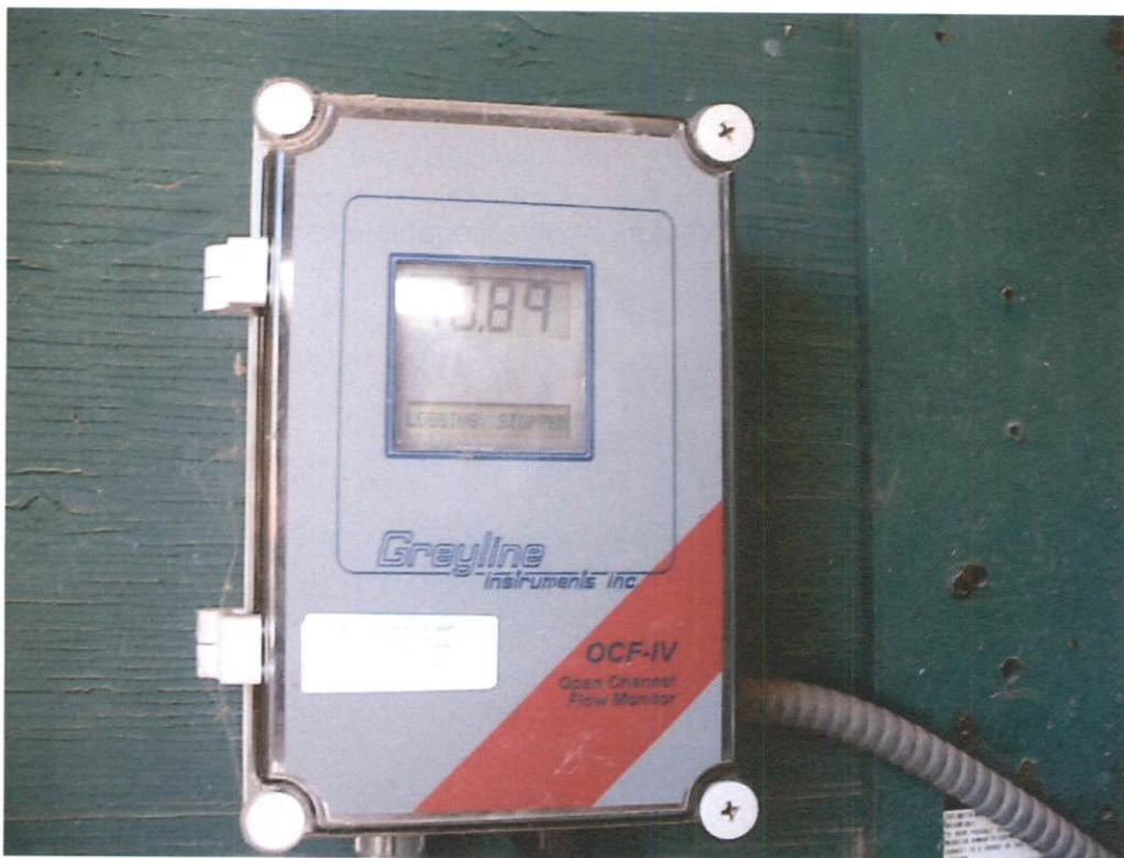
Influent flow meter.
