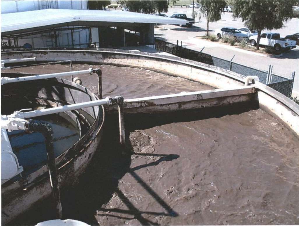
Activated sludge (extended aeration) section of package plant.
