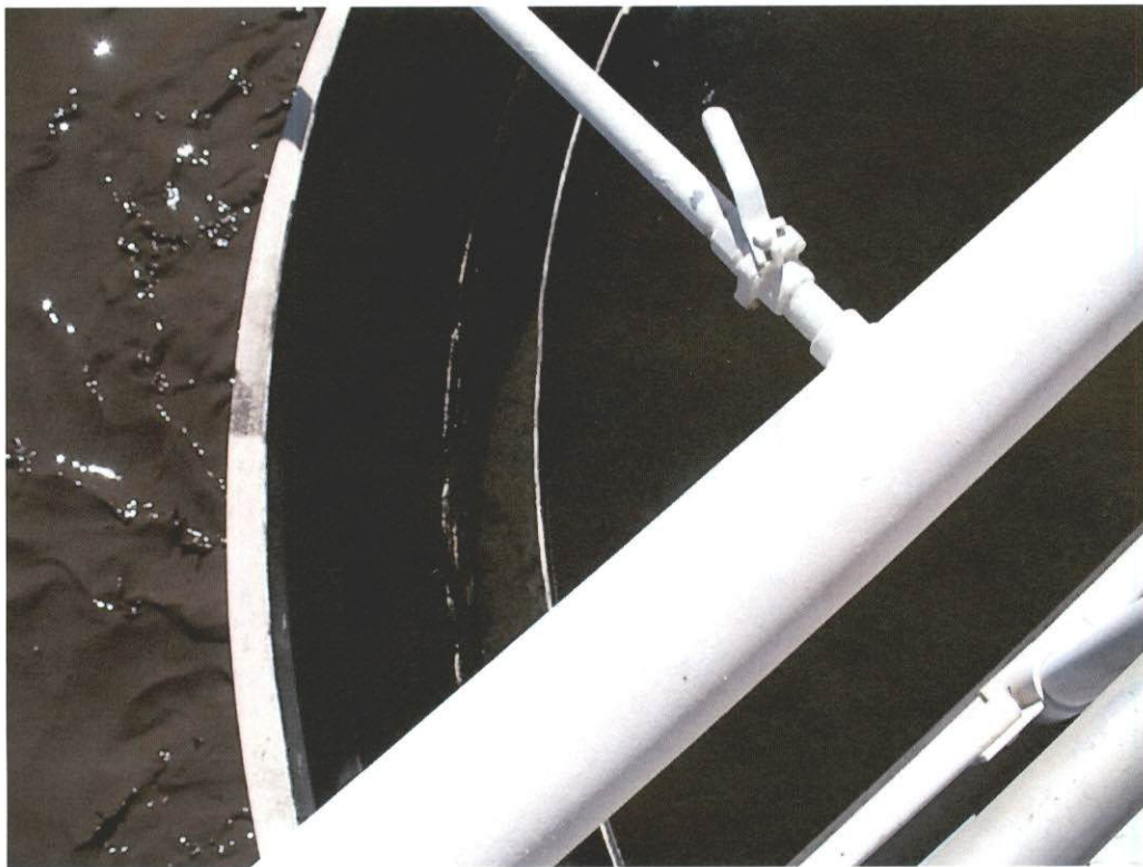
Secondary clarifier section of package plant.
