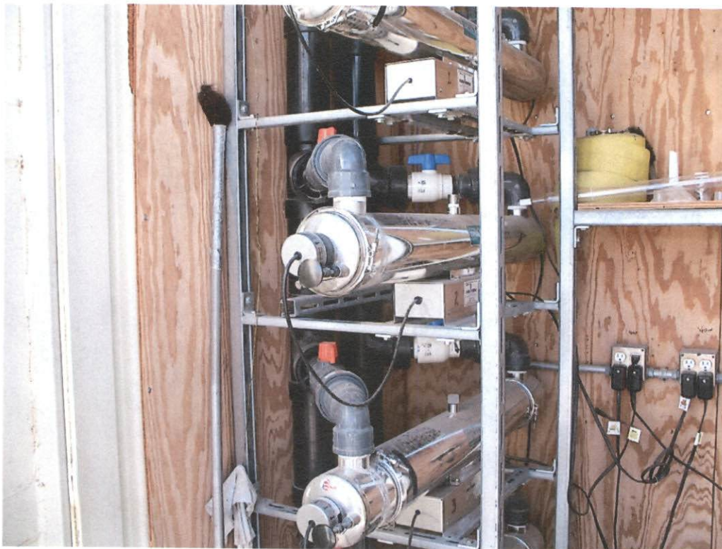
Ultra Violet disinfection banks.
